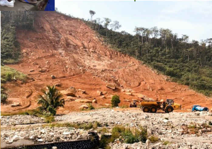
Men at Mudslide area making a path for the water to flow down the hill naturally.
